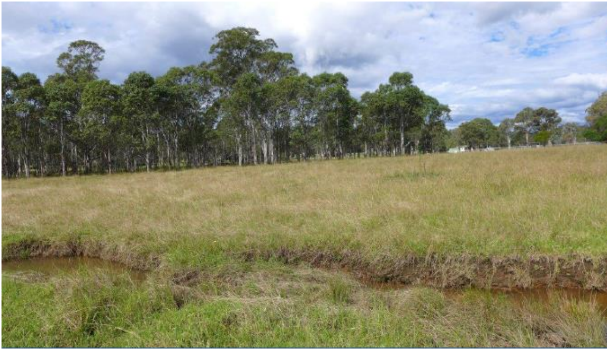
Figure 5. Bank undercutting and slump, lower end of channel
